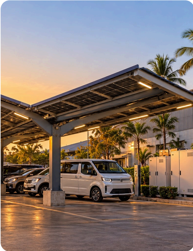
Battery storage for a business site.
